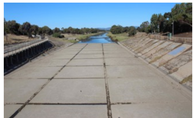
Torrens River Breakout Creek concrete drain presently occupied by free roaming horses polluting the waterway. The NRM Concept Plan is recommending a wetland from Tapleys Hill Road to the Torrens Outlet.
